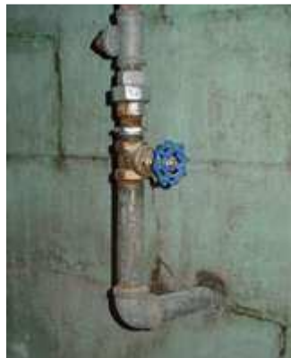
Main water shutoff valve on pipe exiting a basement wall
