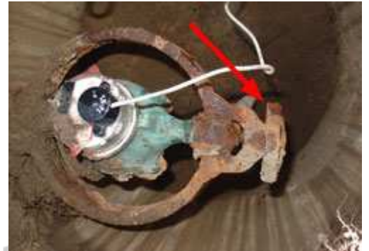
"Hand-turn" water meter shutoff valve.
