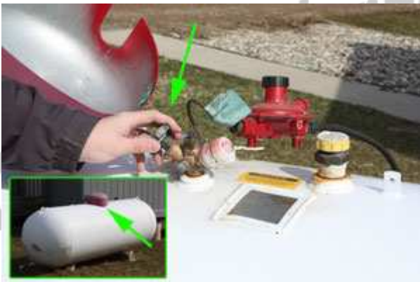
Above ground propane tank shutoff valve example
