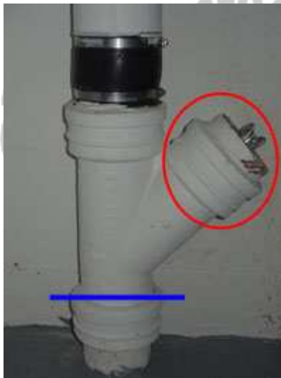
Main sewer cleanout in a house with a basement The top of the test plug should be below the blue line
