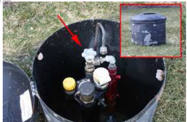
Below ground propane tank shutoff valve example
