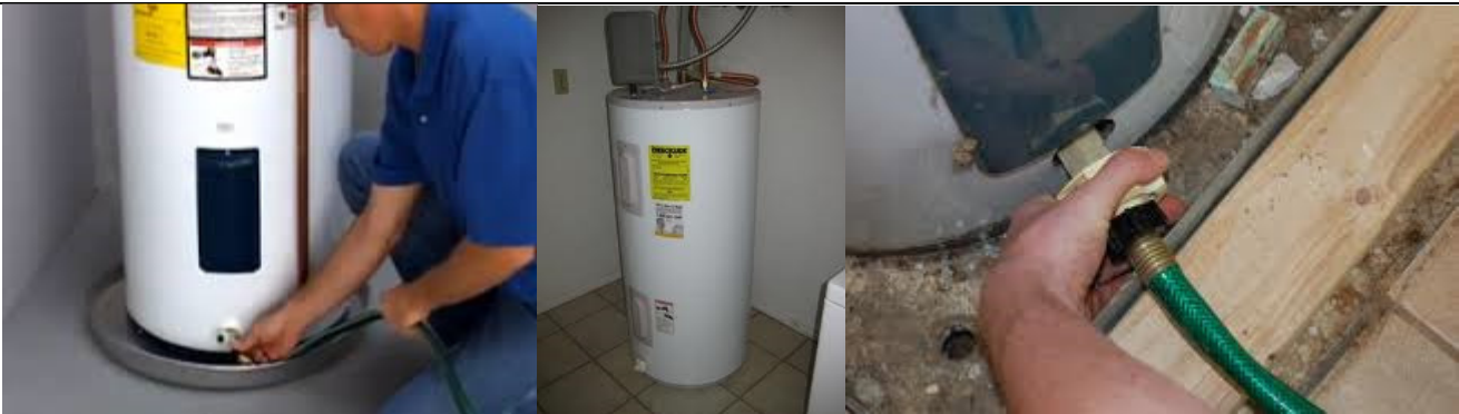
Hot Water Heater
